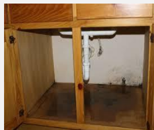
UNDER CABINET LEAKS
